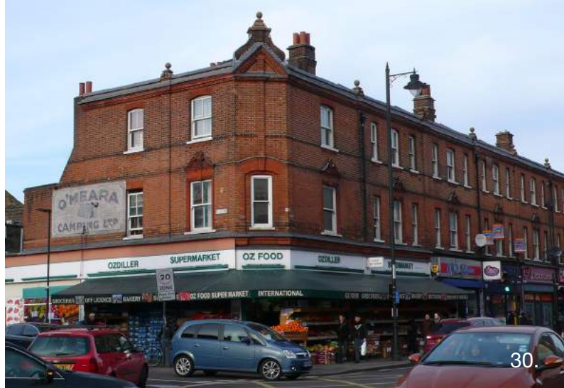
Picture 29. Mosaic Fascia at 479 and 481 High Road, compromising the appearance of Warner Terrace
